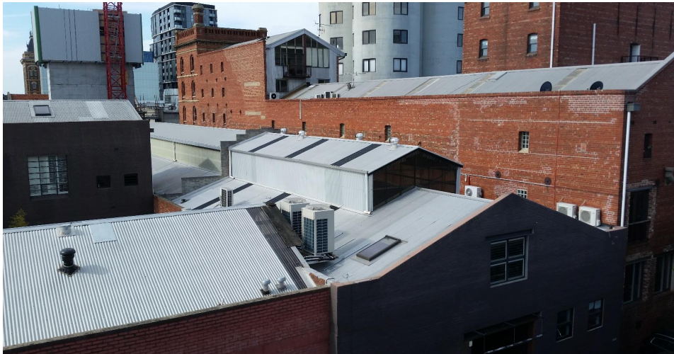
Photo viewed from Care Park car park – Small condensing units serving commercial buildings along western boundary of VDAS site – daytime operation
