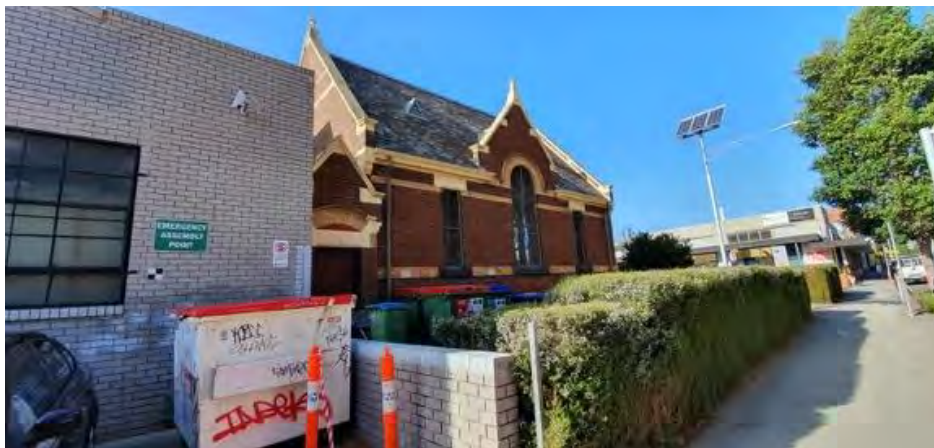
Figure 22. Closer detail of the unsympathetic interface between the heritage place and the projecting neighbouring warehouse. Source: Trethowan Architecture.
