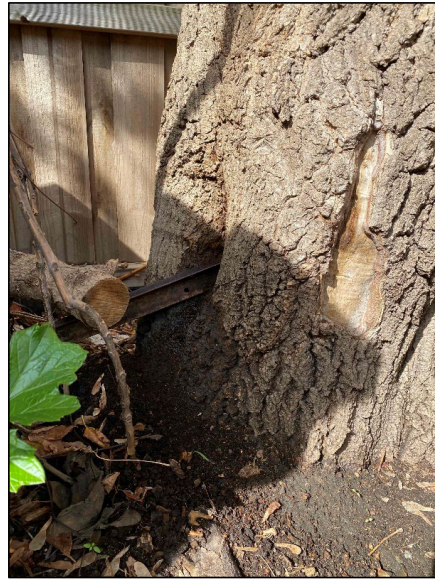
Tree #1, the stem base. A cavity (the steel picket was taken out to inspect the cavity) and a minor wound.
