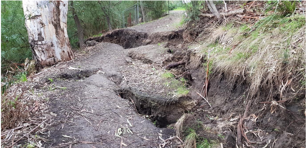
Figure 18. Tree collapse site
