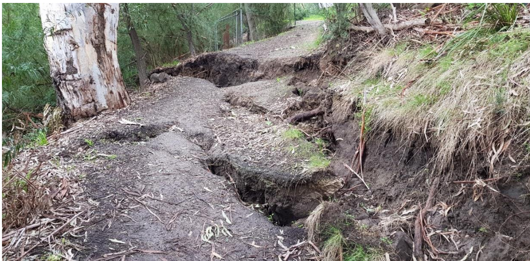
Figure 11: Tree (T1) and bank slump site visit by Alluvium
