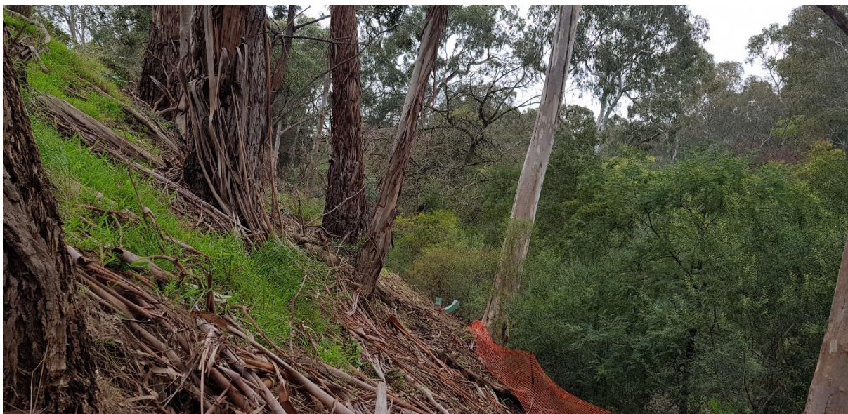
Figure 9: Planted trees on embankment - Trees on the embankment are 20+ year old non-indigenous natives. The trees on the embankment are growing at different angles to each other. Investigate for slumping or ground heaving to determine stability of the trees.
