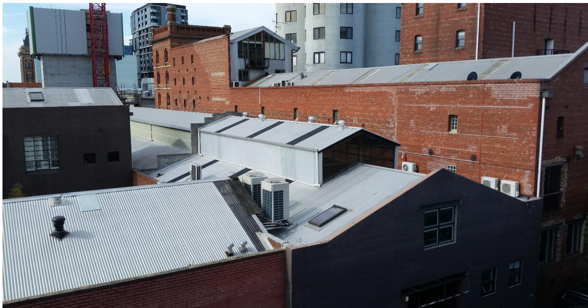
Photo viewed from Care Park car park – Small condensing units serving commercial buildings along western boundary of VDAS site – daytime operation
