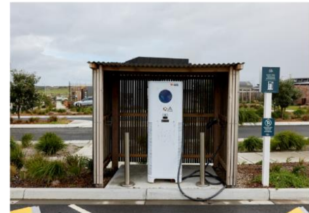
Electric vehicle charging station at The Cape development. Photography by Kim Landy
