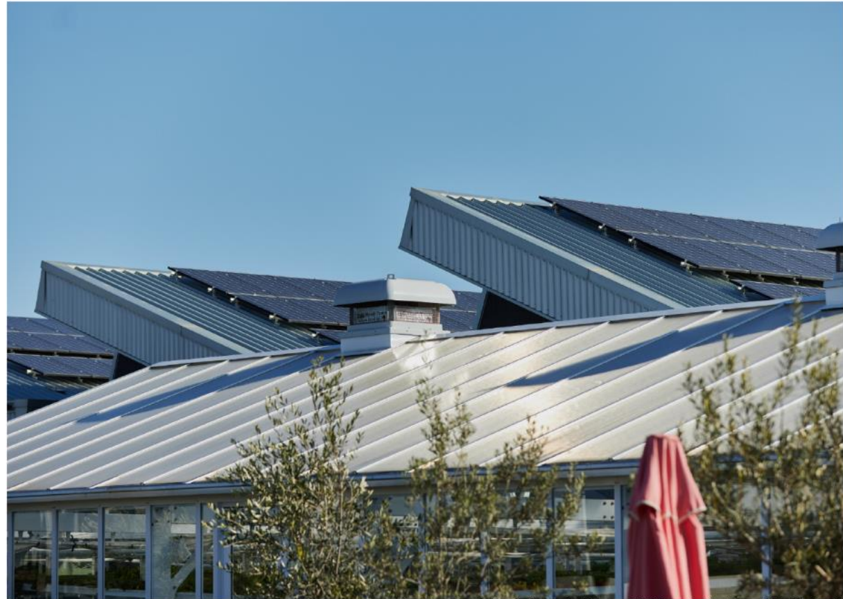
Rooftop solar photovoltaic panels at Burwood Brickworks. Photography by Kim Landy
