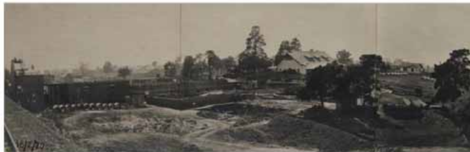
Figure 3 Fairfield Paper mill under construction, February 1920. View looking north-east from the railway line. Source: Amcor Head Office archives.
