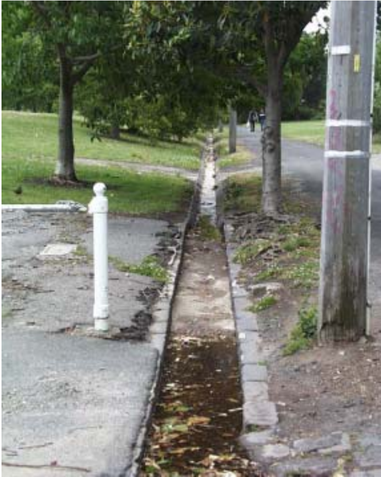
Figure 60 Open drain lined with bluestone pitchers
