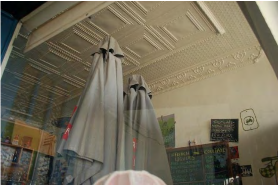
The pressed metal ceiling in No. 67 Smith Street. Proposed grading: Individually significant.
