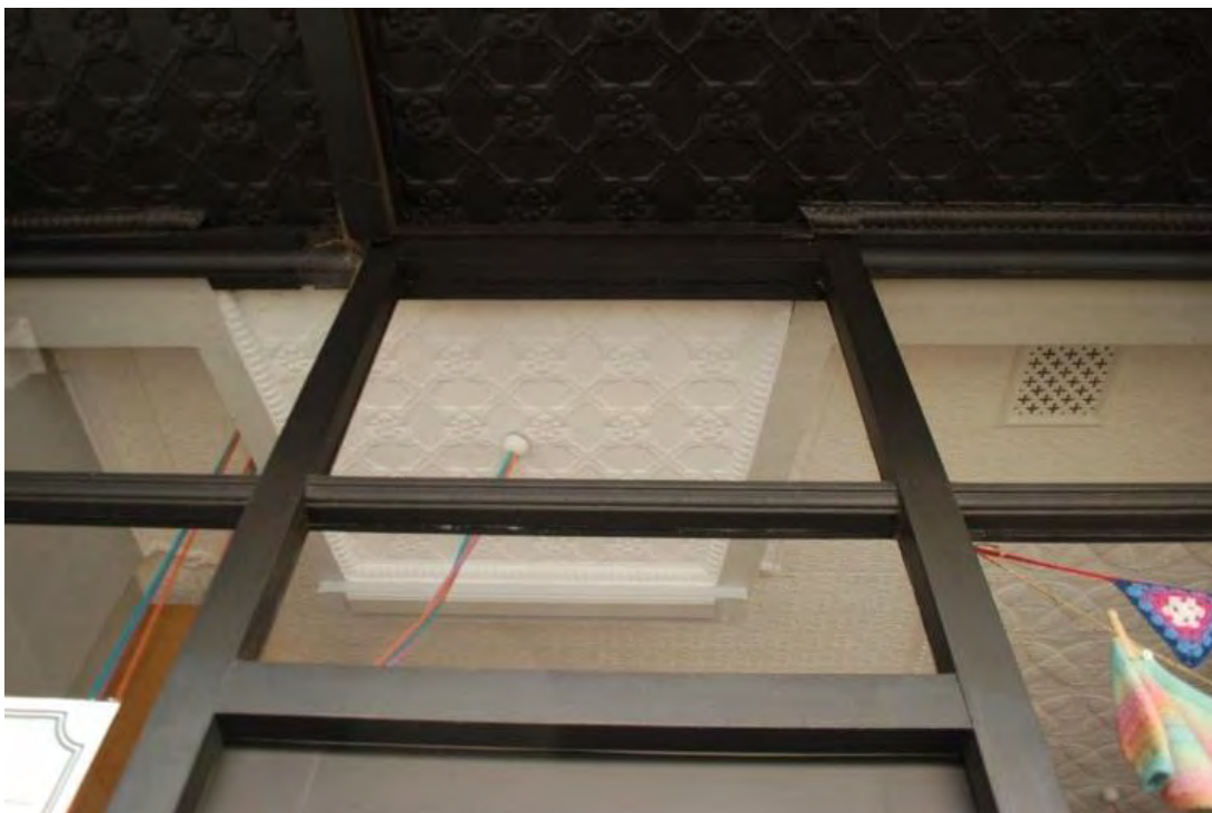
No. 59 Smith Street, Fitzroy. Pressed metal ceiling and original entrance pressed metal soffit which is now contained within the shop. The canopy also has a pressed metal soffit. Proposed grading: Individually significant.
