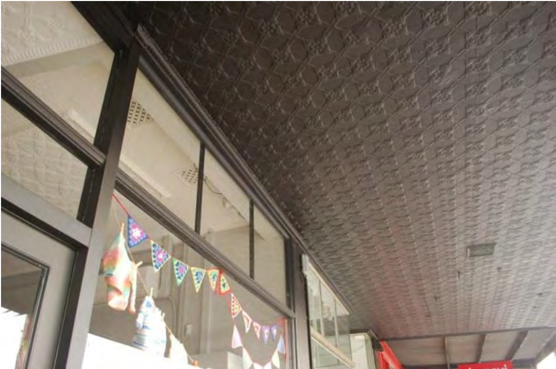
Nos. 59 – 61 Smith Street, Fitzroy. Pressed metal soffit to the canopy and some of the remnant elaborate detailing of the shopfront. Proposed grading: Individually significant.
