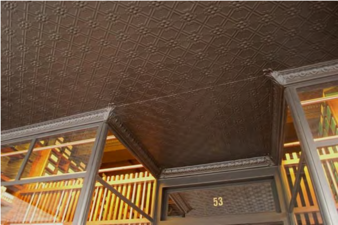
No. 53 Smith Street, Fitzroy. Pressed metal soffit to the canopy and some details of the intact and unusually ornate shopfront. Proposed grading: Individually significant.
